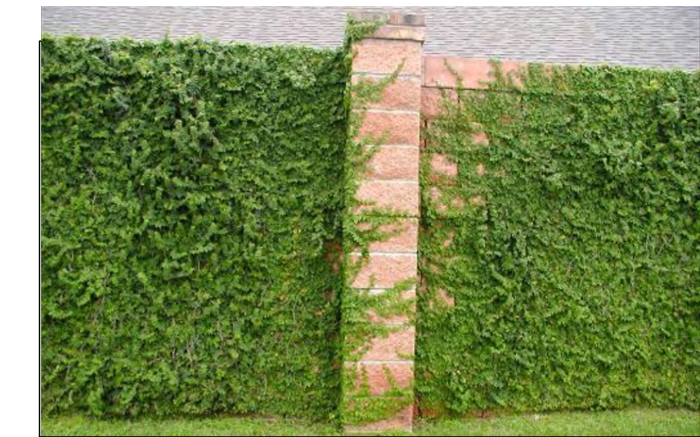
(N) CMU Retaining Wall/Screen, Wall Color to Match Stucco, Plant Vines at Base
