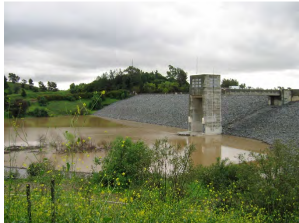
The Brea Dam in Fullerton with the basin partially filled. Image from Fullerton Walks.
