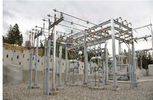
Electrical substations are vital facilities to ensure that electrical service is safe and reliable. Image from Paul Chernikhowsky.
