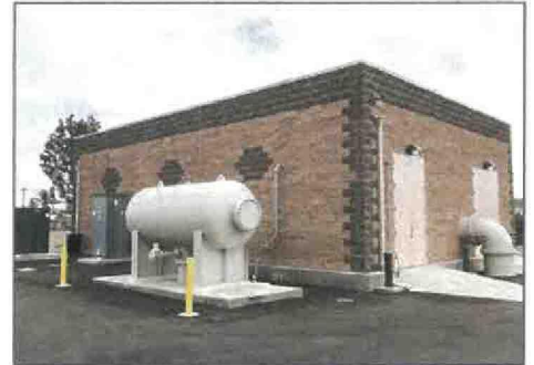
La Palma Water Complex City of Anaheim
